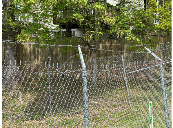
Damaged barbed wire at detention pond fence
