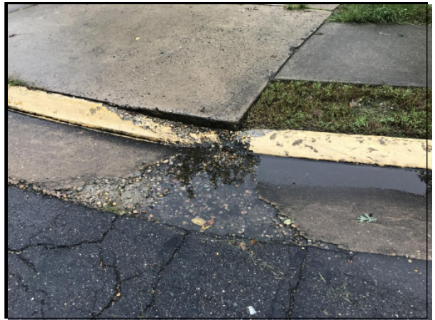
Damage at concrete curbing - Eaton Ct.
