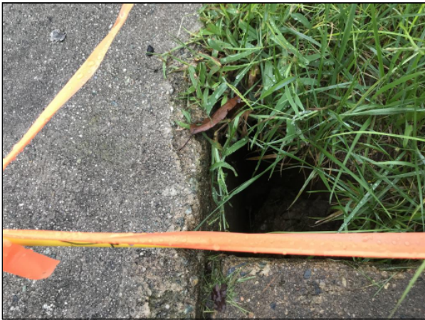
Hole present next to storm drain - Bludridge Ct.
