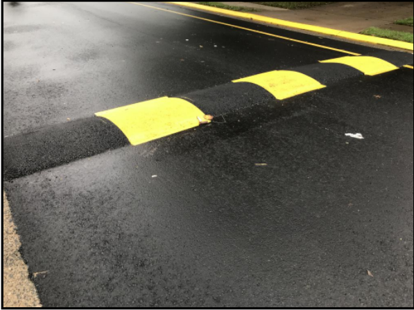
Typical condition of recently resurfaced asphalt surfaces
